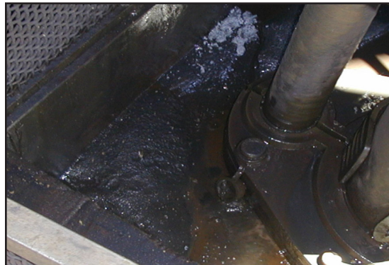
Pre-existing condition of concrete
