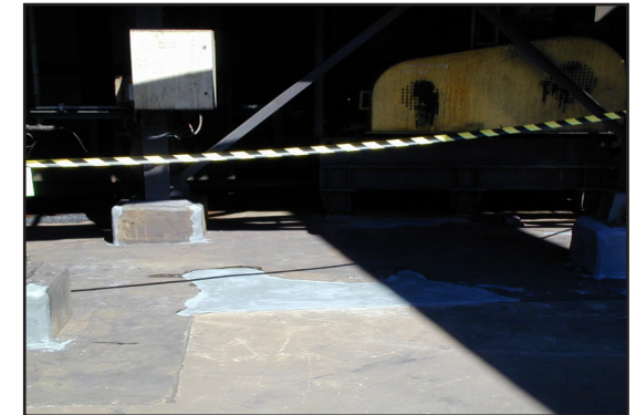
ARC coated surfaces with minimal repairs indicated in 2010
